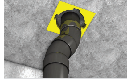
Installed pipe through FCID device
